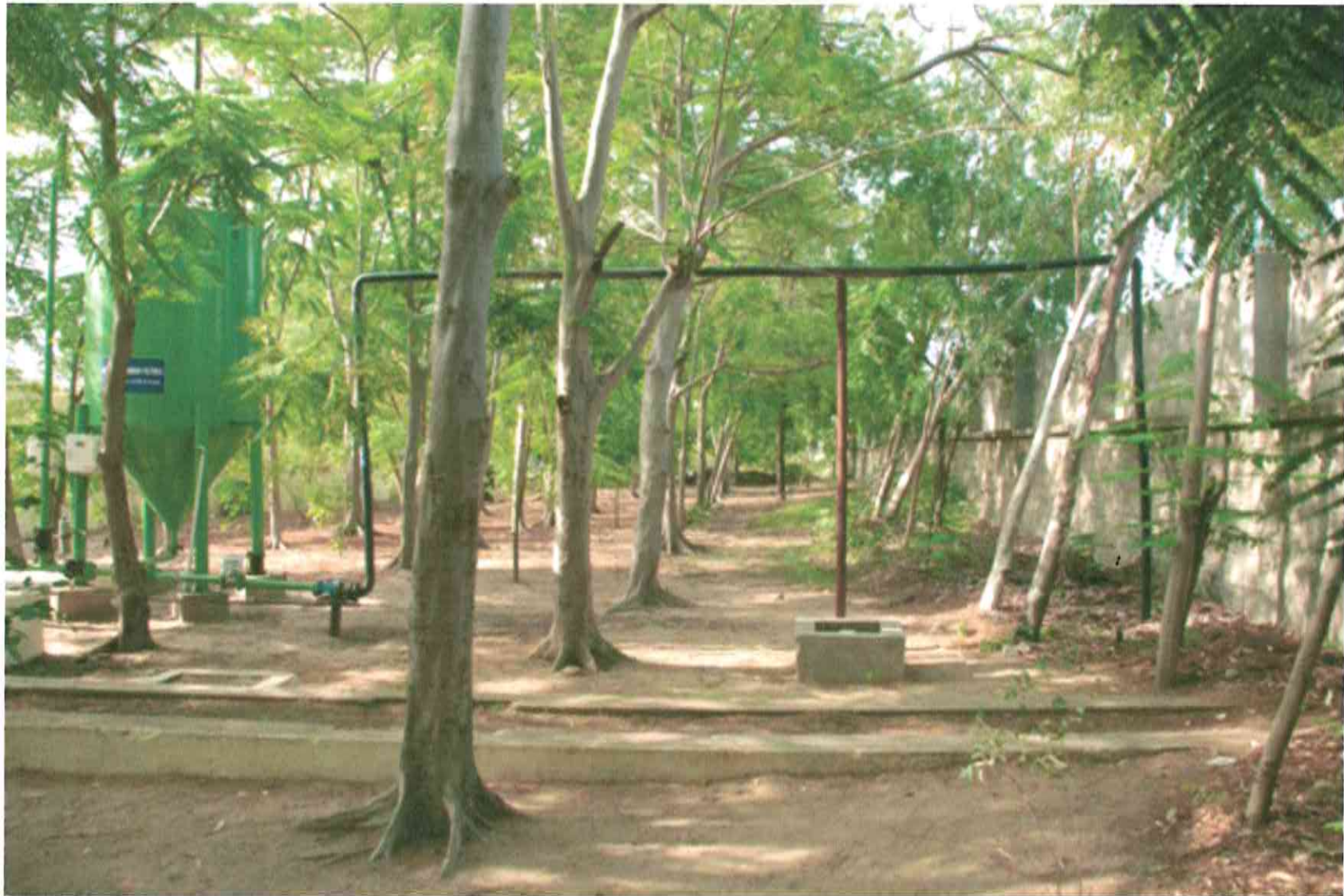
Greenery in ETP - rear side of Aeration tank.
